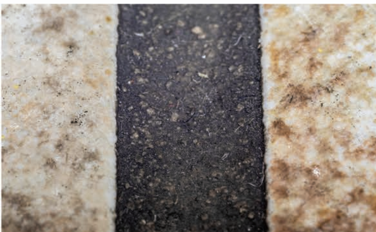
Close up photo of biofilm build-up in a grout line.
